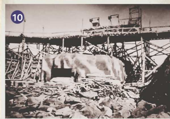
The defences under construction at Bibette Head in 1943, showing the completed 10.5cm casemate.
